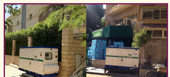
Kirloskar 40kVA generator installed at residential units for Installation for standby power for supermarkets.
