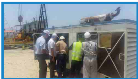
Inspecting the generator during the service campaign
