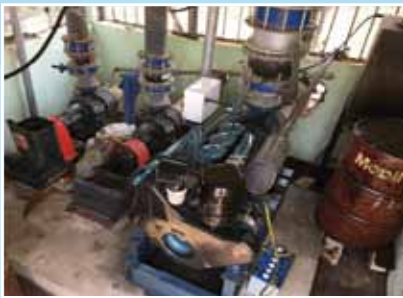
Kirloskar Pumpset in operation
