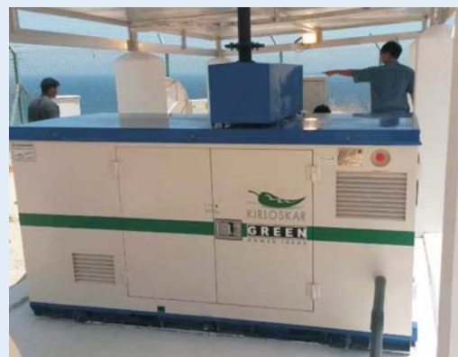
Kirloskar Genset At Omantel
