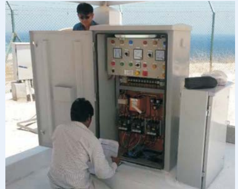
Commissioning in Progress
