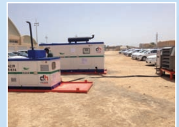
15KVA & 160KVA Generator Connected to Load Bank for demonstration
