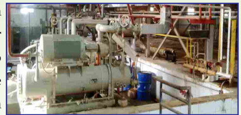
1 st XRV screw compressor package installed in Saudi Arabia
