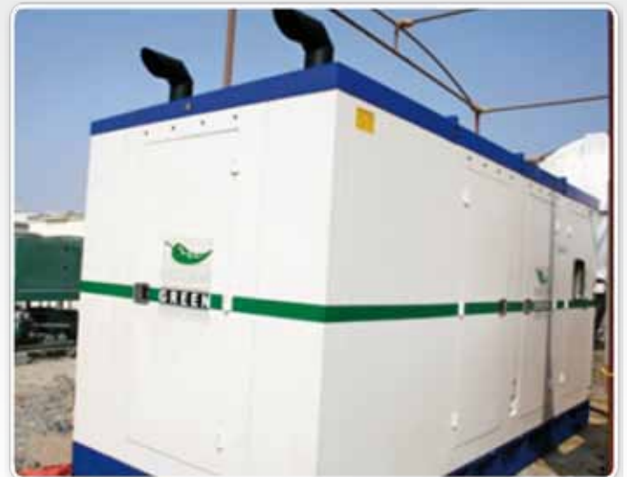
400kVA installed at Ras Al Khaimah – 24x7 operation.
