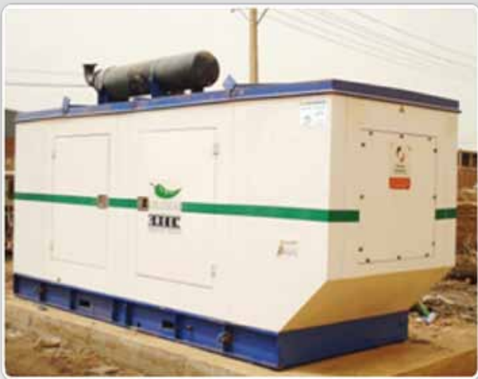
A Kirloskar 160kVA generating set powers a complete green house project near Khartoum, Sudan.
