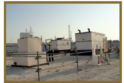
Generating Sets installed at L&T site
